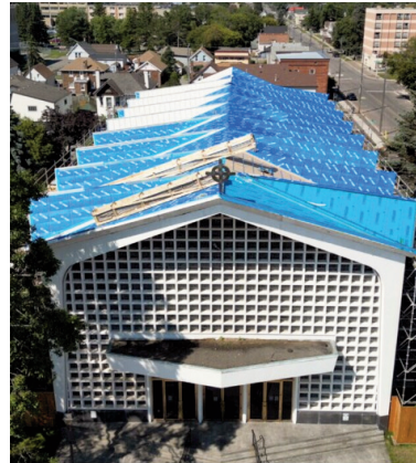
NEW ROOF: Contractors have made good progress on the new roof for the iconic St. Patrick's Cathedral.
