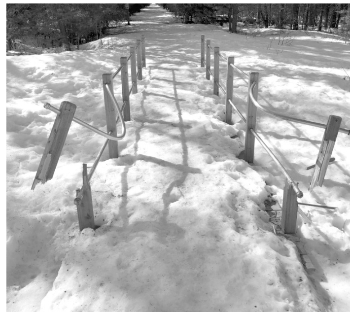
VANDALIZED: A bridge in the Mills Block Forest has been damaged by a vehicle.
