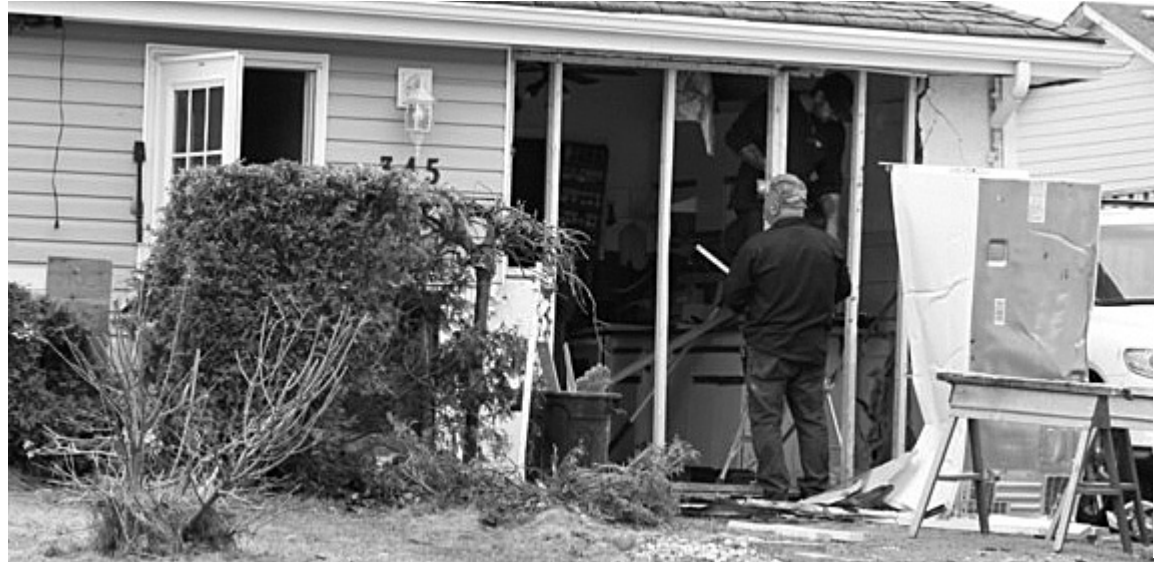
RUDE AWAKENING: Repairs are made on Saturday morning to a home on County Boulevard after a minivan crashed into it earlier.
