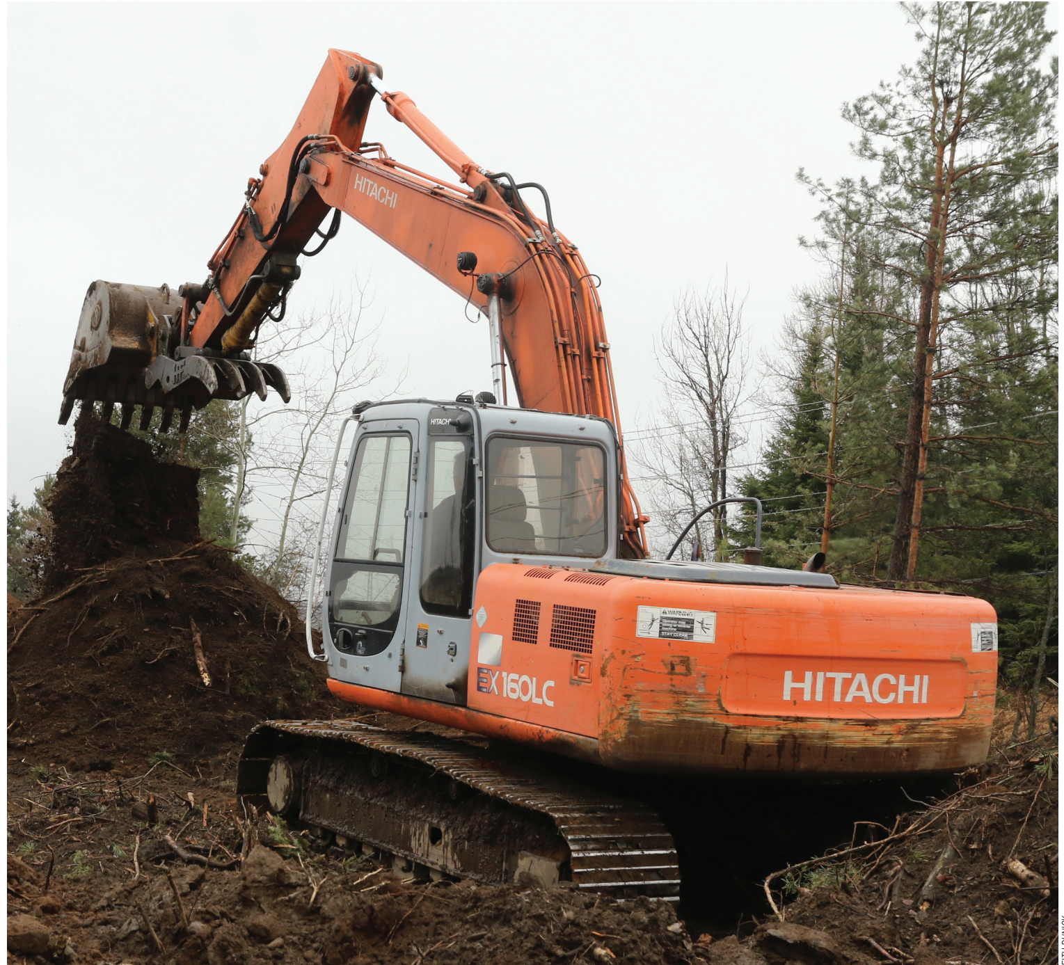
READY, SET, GO: Site work for a planned two-dome indoor soccer complex is nearing completion and construction is expected to begin shortly, according to the developers.
