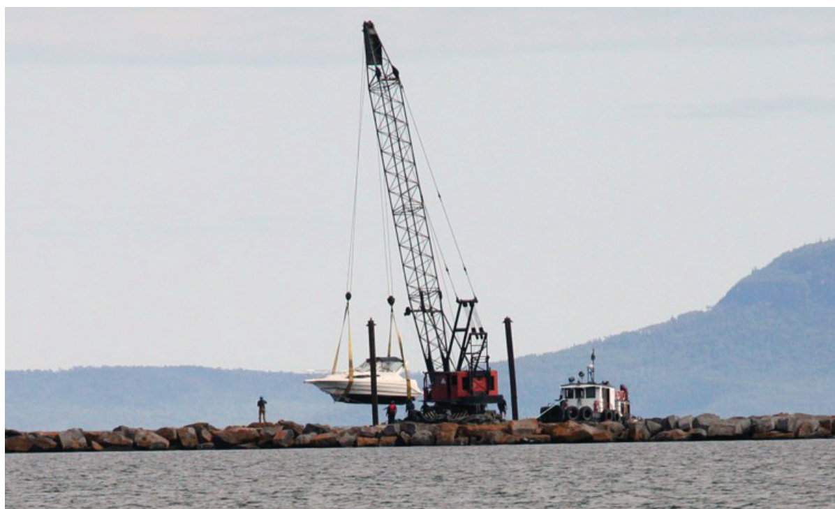
A crane was used to remove a boat that crashed into the breakwall in Thunder Bay Harbour on Aug. 22, 2019. (FILE)
