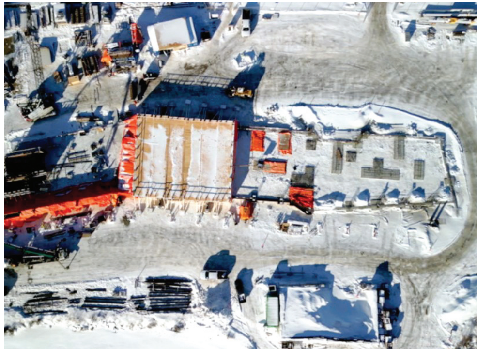
Construction work has begun on the waterfront Thunder Bay Art Gallery project. (Blair Wright)
