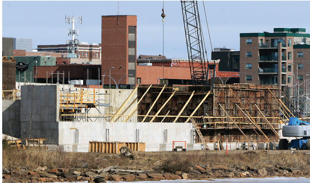
The Thunder Bay Art Gallery's new waterfront home is under construction and expected to open in 2025. (Leith Dunick)
