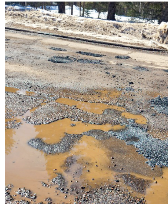
Potholes like these on Farrand Street can be found all over.
