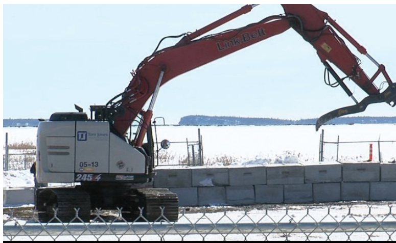
Crews are set and equipment is ready to start work on the new art gallery. (Mike Lang/TBT)
