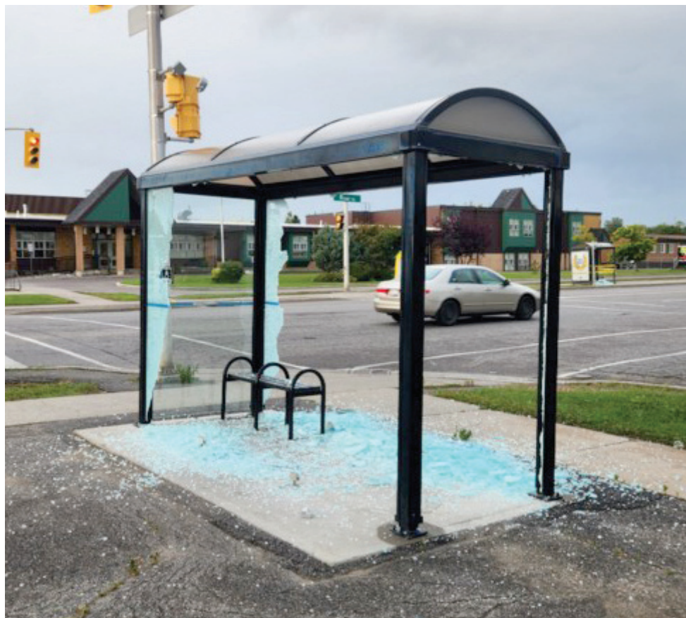
This bus shelter along River Street was damaged by a vandalism attack over the weekend.
