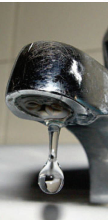
CAUSING LEAKS?: The city will stop using sodium hydroxide in its water supply.
