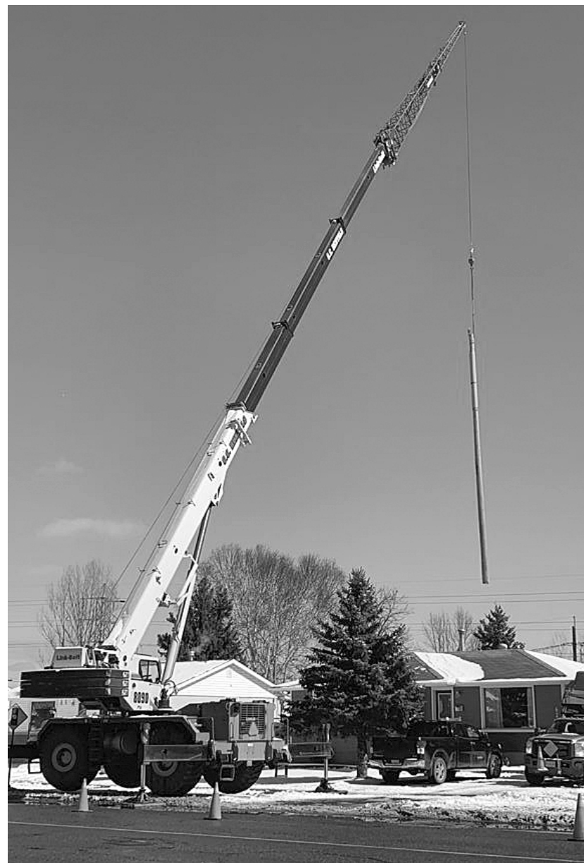
IN THE AIR TONIGHT: Synergy North crews last Thursday install a hydro pole behind an Edward Street home.
