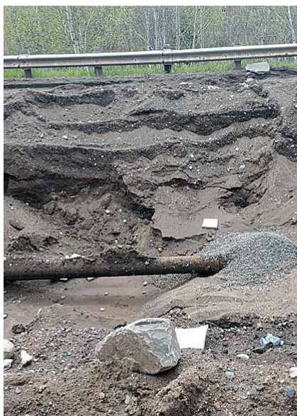
Work continues on a sinkhole on River Street that has closed the road for several weeks. (Gary Rinne)
