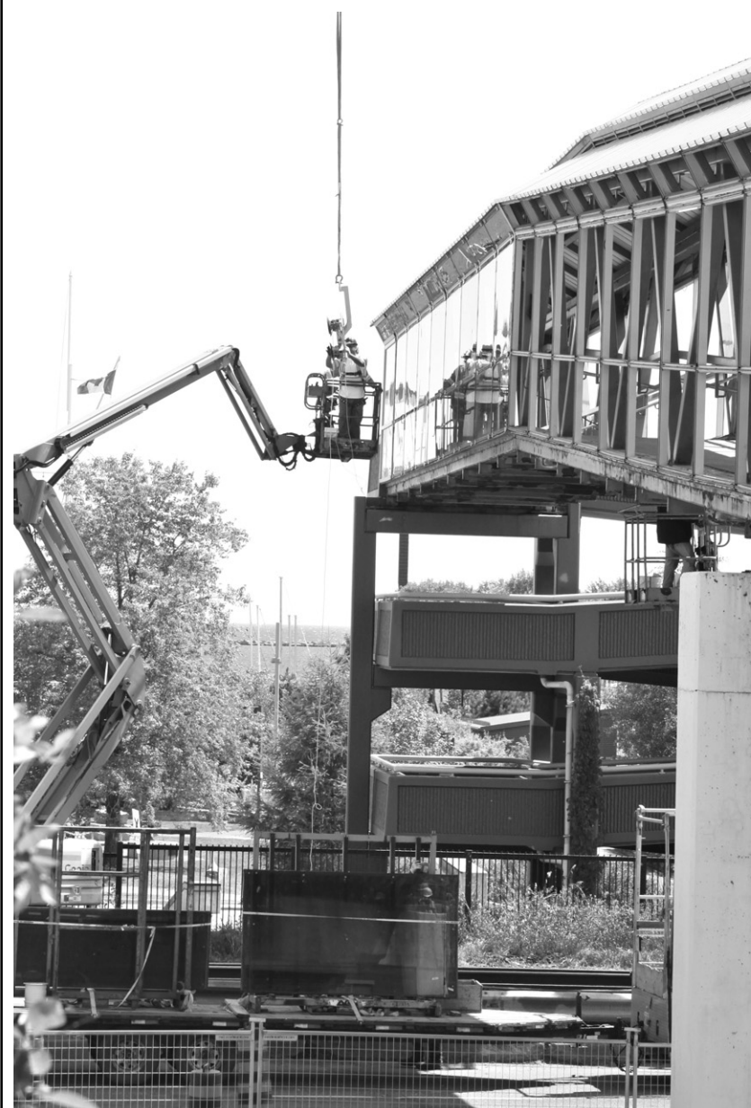
GONE FOR REPAIR Workers with Tom Jones Corp. removed one of two sections of the Marina Park pedestrian overpass last Thursday.
